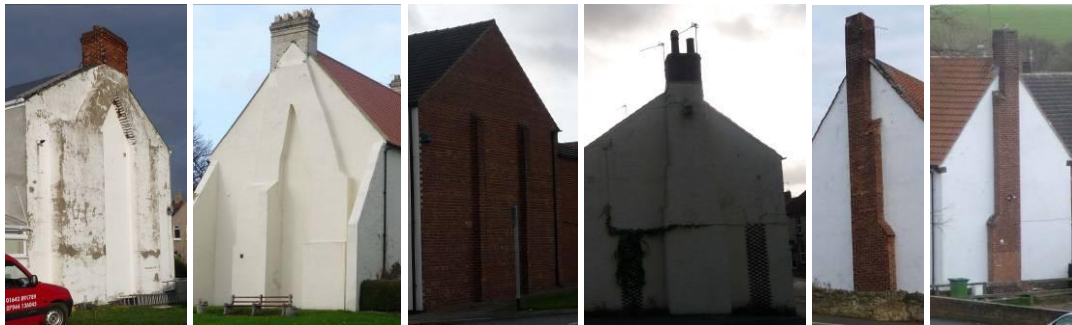
Plate 24. Partial demolition explains the presence of a number of external chimney stacks and buttresses (i, ii, iii) but they have also been incorporated into new build or added to older properties.
