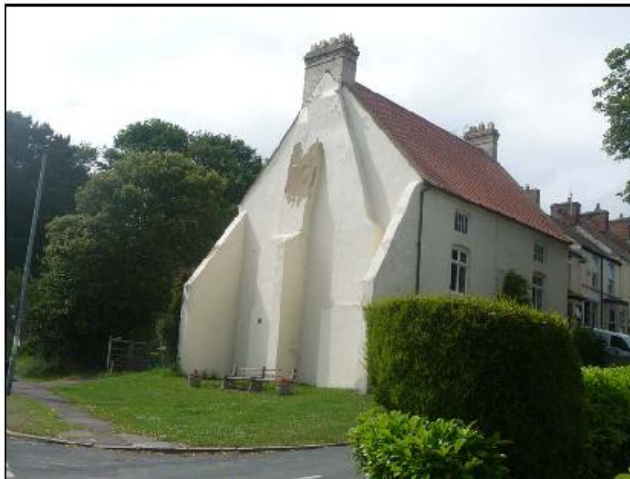
The Old Manor House has lost two bays to road widening (hence the buttress) and has lost its traditional multi-pane windows to first floor level. The roofing materials have changed and the stone detailing around the windows has been covered with render.
